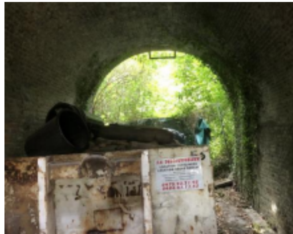
Conteneur obstruant le tunnel
